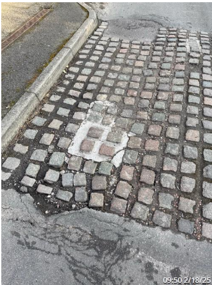
Figure 9 - Granite setts and rutting, Station Rd
