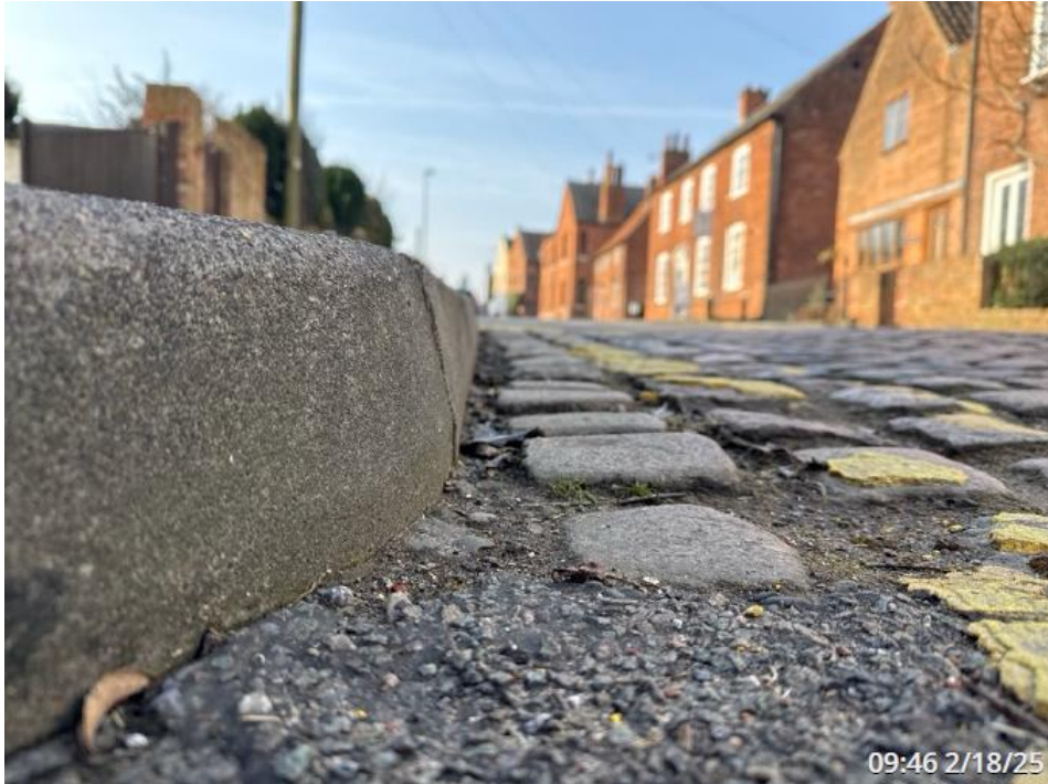
Figure 8 - Kerb upstand relative to sunken speed hump profile, Station Rd
