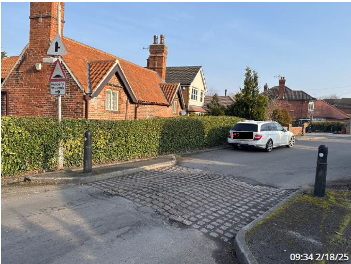
Figure 5 - Speed hump condition, Station Rd
